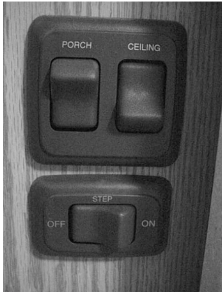
Entry Switch Panel
