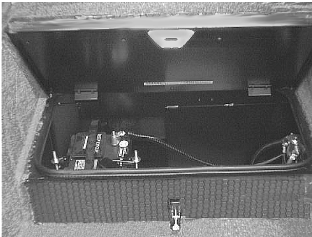
House Battery Storage in Entrance Step Models 24F, & 24V, 27L, 29B & 31C/T
