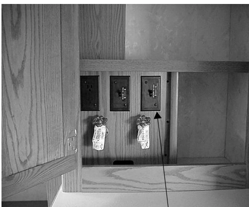
Engine Block Heater Switch (Typical)
