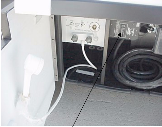
Inverter Charger Unit Location
