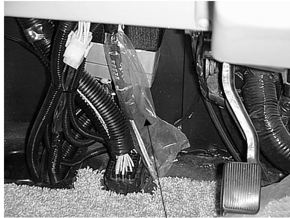
CB Wires (in plastic sheath)
