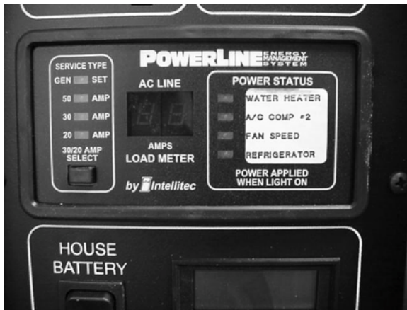
EMS Display on OnePlace Monitor Panel
