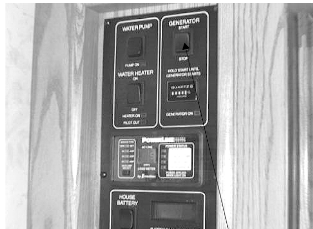
Generator Switch and Hourmeter
