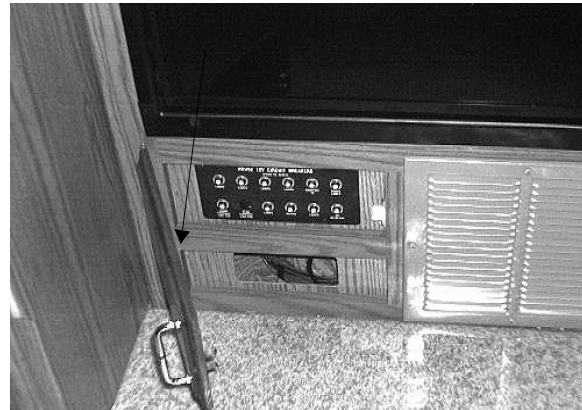
House 12-Volt Circuit Breaker Panel
