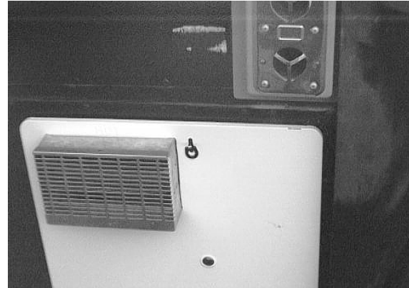
Water Heater Service Access Panel
