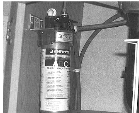
Water Filter Assembly - Below Galley Sink
