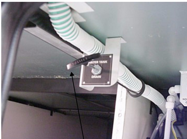
Water Tank Drain Valve (pull to open)
