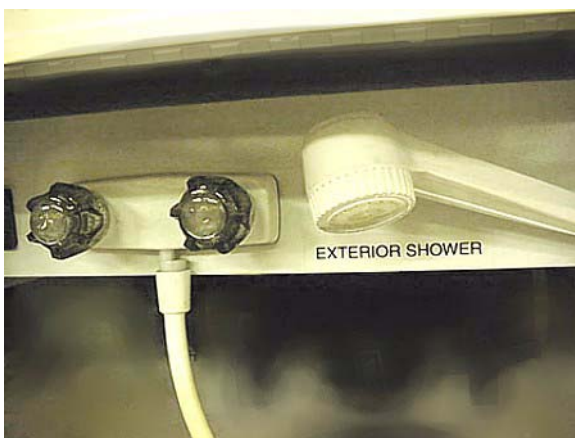
Exterior Shower/Wash Station (Typical)
