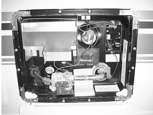
Water Heater Exterior Service Access
