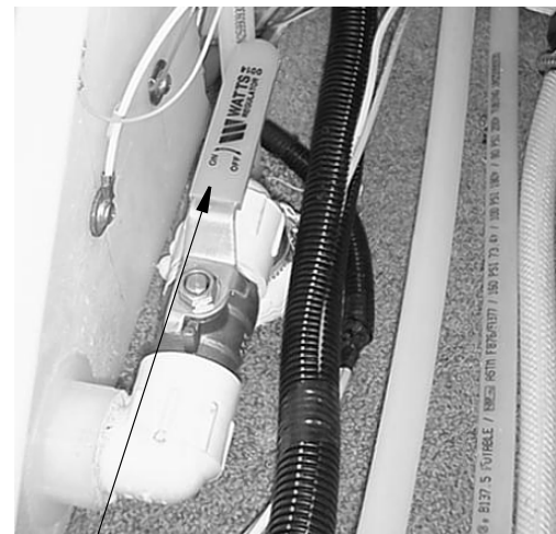
Water Tank Drain Valve
