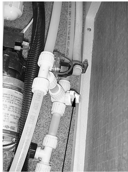
Waterline Drain Valve (Typical)
