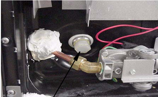
Water Heater Drain Plug Remove with socket
