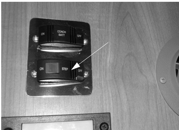
Entry Step Switch (Located near entrance door)
