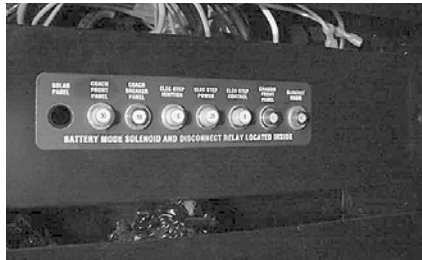
Chassis and House 12V Breakers (cover off)
