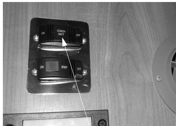
Aux. Batt. Switch - Typical (Located near entrance door)
