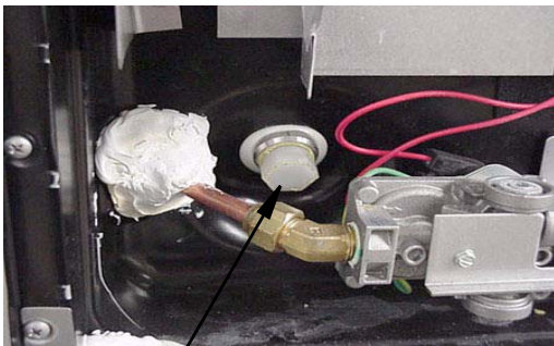
Water Heater Drain Plug Remove with socket.
