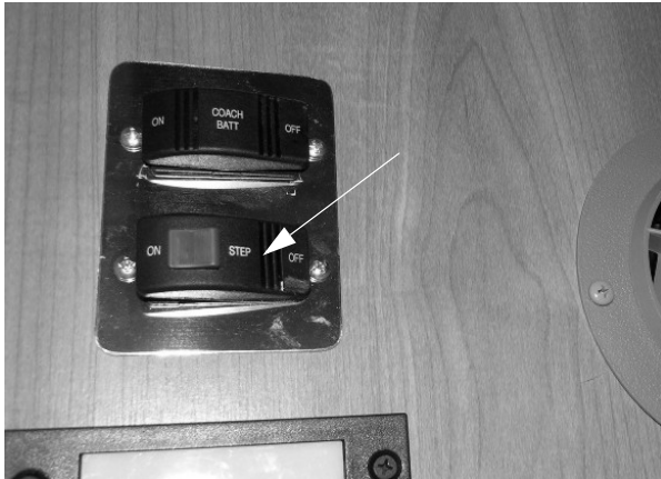
Entry Step Switch (Located near entrance door)
