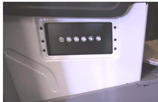
Chassis and House 12V Breakers on side of passenger seat base toward door (shown w/cover off)
