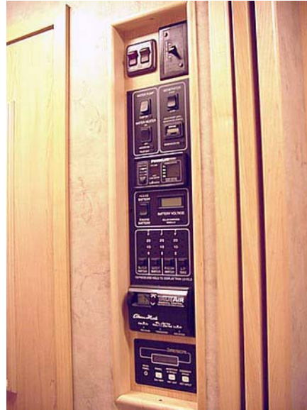
OnePlace Monitor Panel -Typical View
