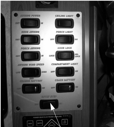
Entry Step Switch (Located near the entrance door) -Typical View
