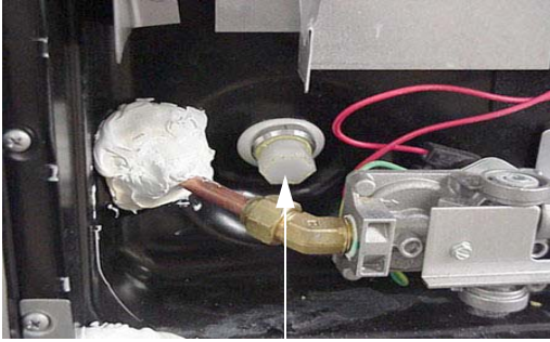
Water Heater Drain Plug (Remove with socket)
