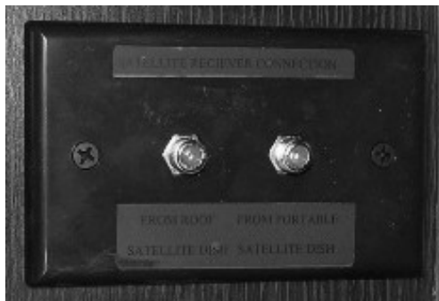
Interior Connection for Satellite Dishes (Located in cabinet near TV) - Typical View
