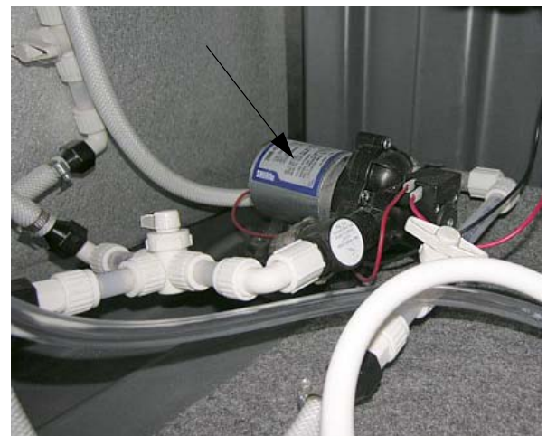
Water Pump -Typical View
