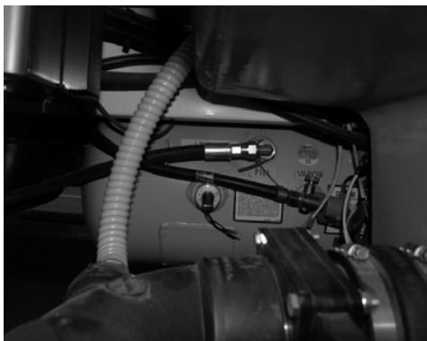
Propane Gas Tank (Located underneath of coach) -Typical View
