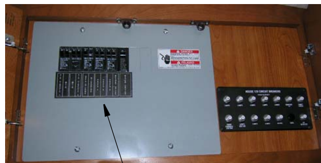
House 120-Volt AC Circuit Breaker Panel
