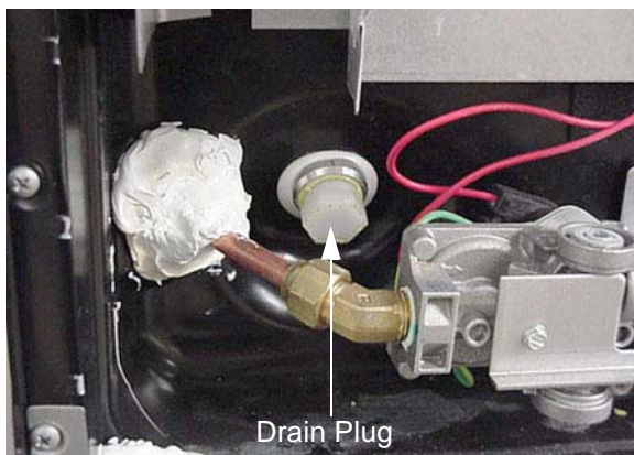
Water Heater Service Access -Typical View
