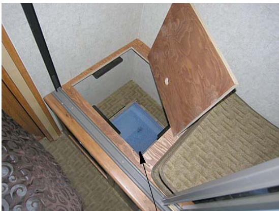
AC/Furnace Filter under wardrobe floor panel
