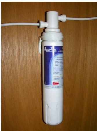
Water Filter Assembly (Located below galley sink)
