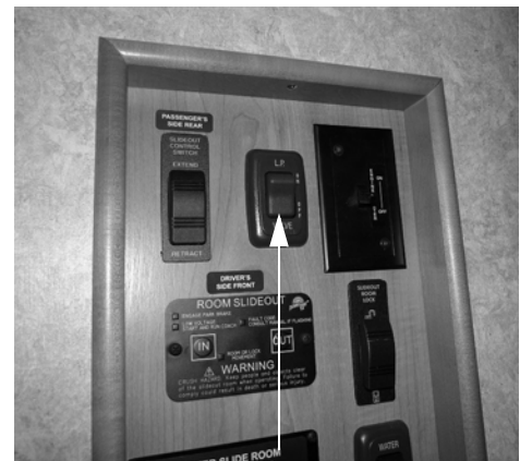
Main Tank Valve Switch (Located near monitor panel area) -Typical View
