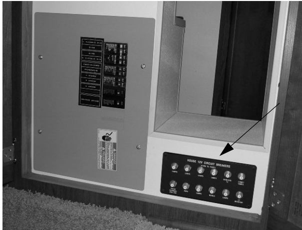
House 12V Circuit Breaker Panel -Typical View
