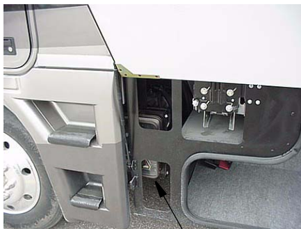
Hydraulic Pump Access (Open storage compartment door behind driver's side front tire)
