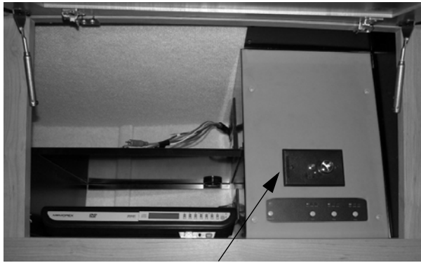
TV Signal Amplifier Power Switch (Typical View)
