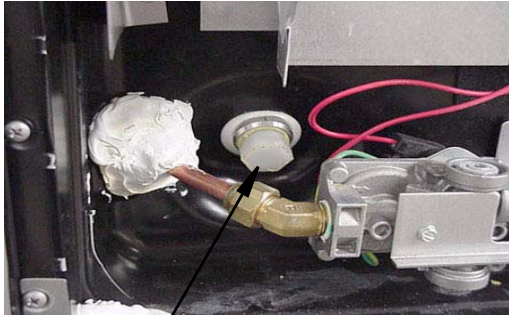
Water Heater Drain Plug Remove with socket
