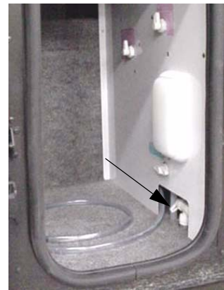
Waterline Drain Valve -Typical View
