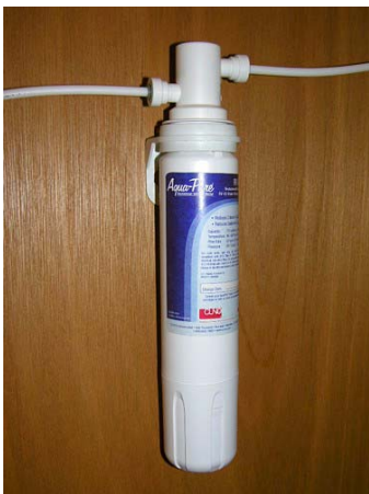
Water Filter Assembly below Galley Sink
