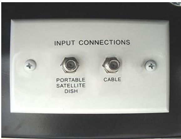
Exterior Connection for Satellite Dish and Cable TV (in the Shoreline Compartment)
