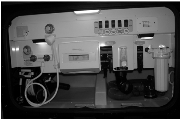
Water Service Center - Typical View
