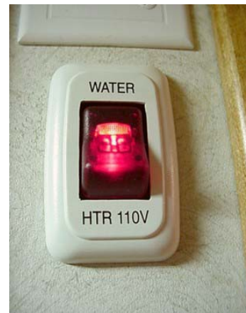
Electric Water Heater Switch (Located near monitor panel)
