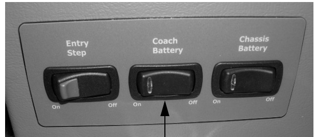
House/Coach Battery Disconnect Switch (Located near entrance door) -Typical View
