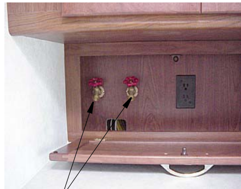
Water Supply Faucets - Typical View
