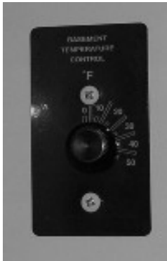
Basement Temperature Control
