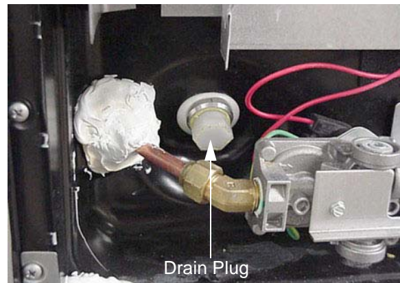
Water Heater Service Access -Typical View
