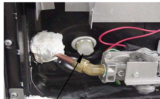
Water Heater Drain Plug (Remove with socket)
