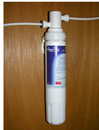
Water Filter Assembly (Located below galley sink)
