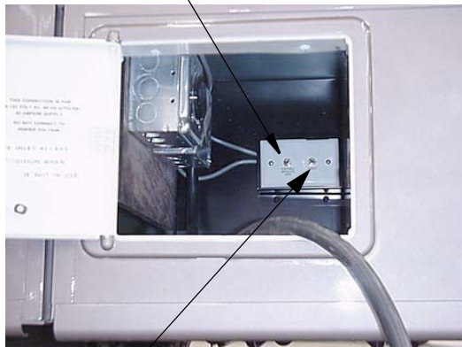
Portable Satellite Dish Connection
