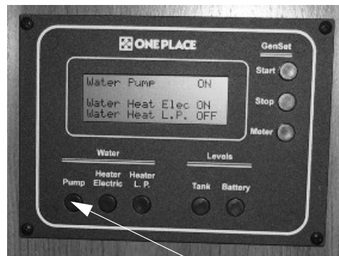
Water Pump Switch
