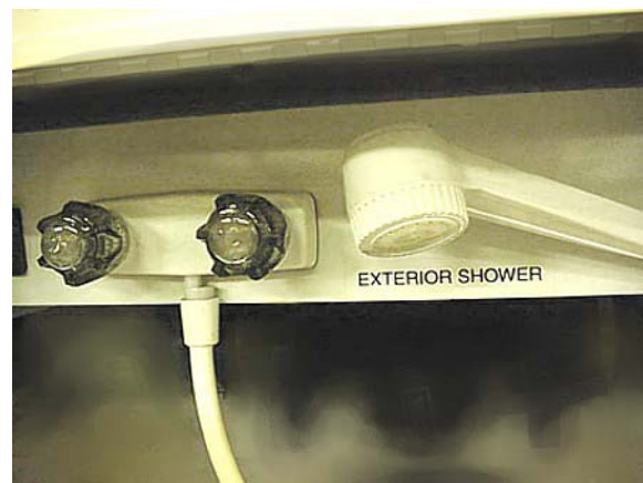
Exterior Shower/Wash Station -Typical View
