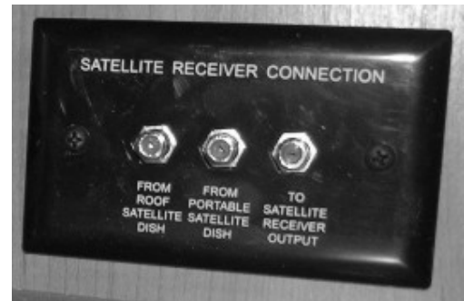
Interior Connection for Satellite Dish (Located in cabinet near TV) -Typical View
