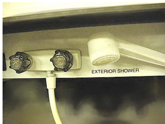
Exterior Shower/Wash Station -Typical View
