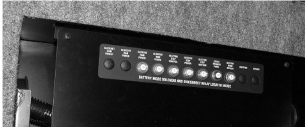
Chassis and House 12V Breakers (Located in passenger side compartment) -Typical View * Shown with cover removed
