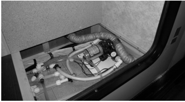
Water Pump (Located beneath removable access panel in passenger rear compartment) -Model 24K Shown
