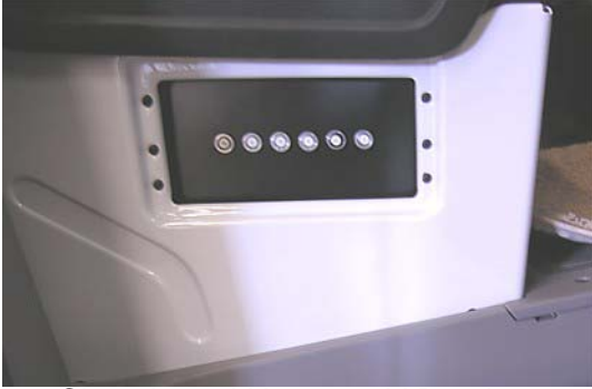
Chassis and House 12V Breakers (Located on side of passenger seat base toward door) * Shown with cover removed -Typical View
