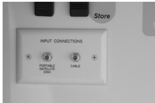
Exterior Connections for Satellite Dish and Cable TV (Located in water service center) -Typical View
