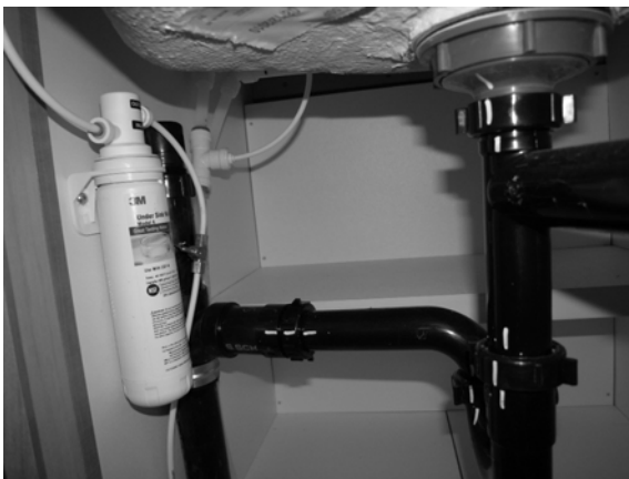
Ice Maker Water Filter Assembly (Located below galley sink)
