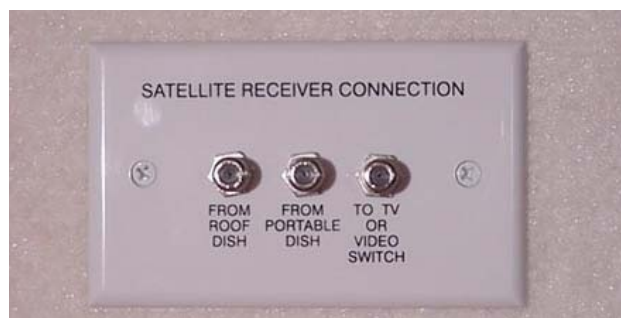
Interior Connection for Satellite Dish (Located in cabinet near TV) -Typical View
