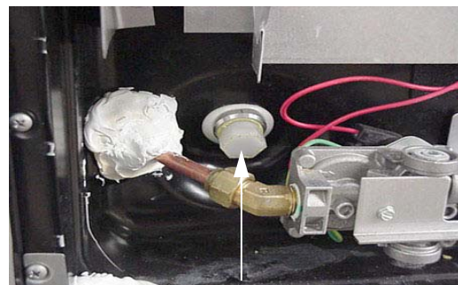
Water Heater Drain Plug (Remove with socket)
