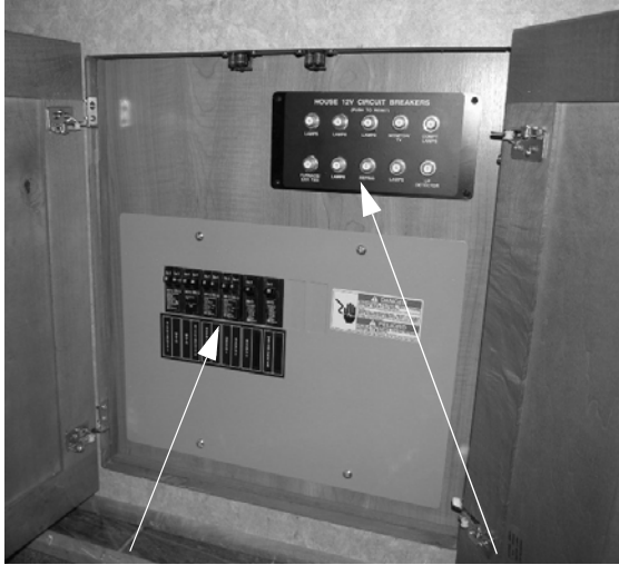
120-Volt House Circuit Breakers
