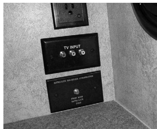
Bedroom DVD/Satellite Receiver Connection -Typical View
