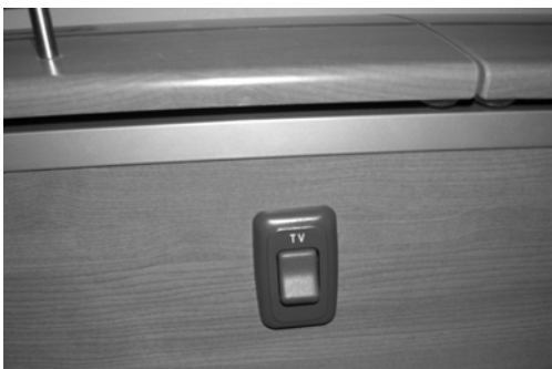
TV 12-Volt Master Power Switch (Located on underside of bedroom overhead cabinet) -Typical View
