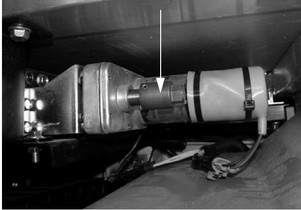
Motor/Gear Assembly (Viewed from inside compartment door opening) -Typical View
