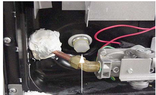
Water Heater Drain Plug (Remove with socket)
