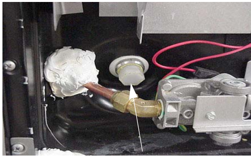
Water Heater Drain Plug (Remove with socket)
