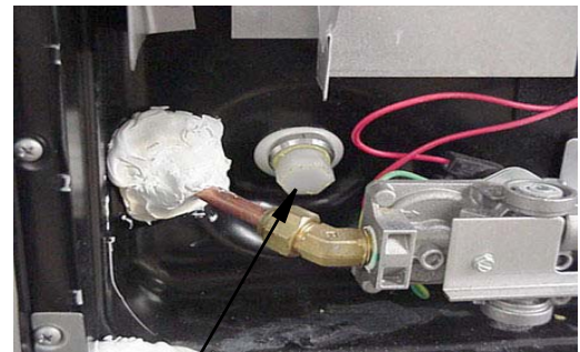
Water Heater Drain Plug (Remove with socket)
