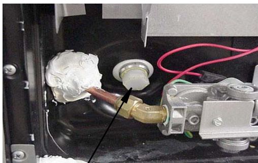
Water Heater Drain Plug (Remove with socket)
