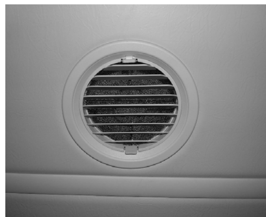
Return Air Vent (Shown with filter installed)
