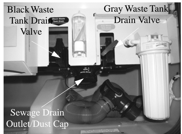
Black and Gray Waste Tank Drain Valves (Located in water service center) * Model 42QD
