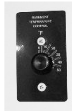
Basement Temperature Control
