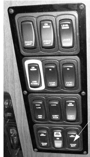
House/Coach Battery Disconnect Switch (Located near entrance door) -Typical View
