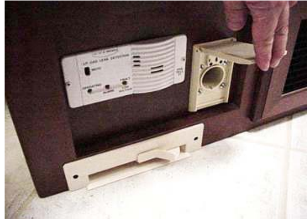
Central Vacuum Cleaner System -Typical View
