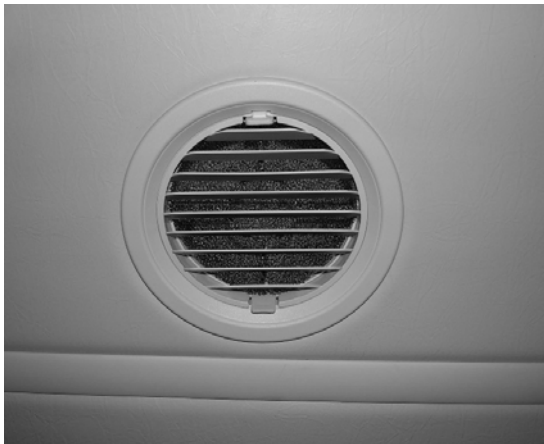
Return Air Vent (Shown with filter installed)
