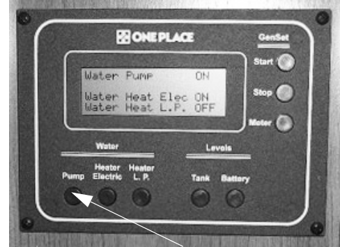
Water Pump Switch
