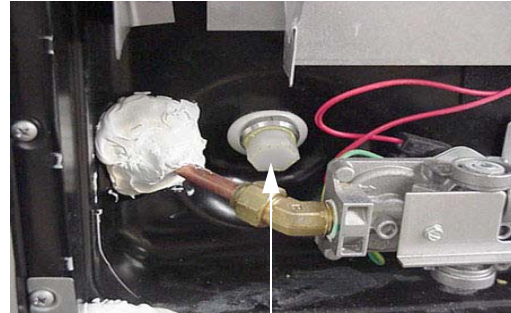
Water Heater Drain Plug (Remove with socket)
