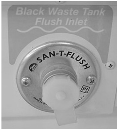
Black Waste Tank Flush Inlet (Located in water service center) -Typical View
