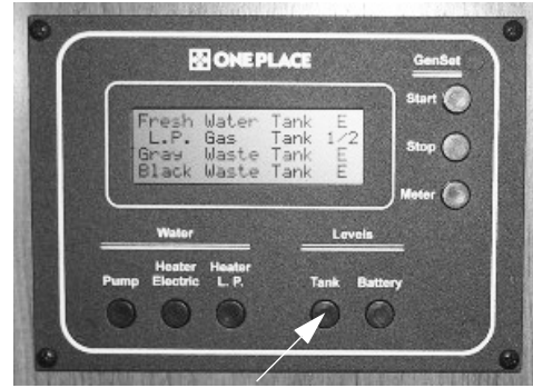
Tank Levels Switch
