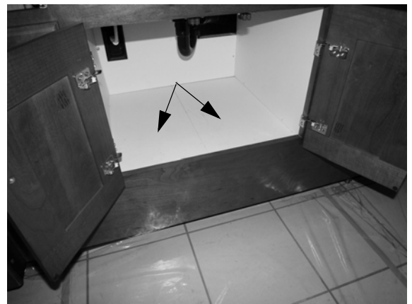
Access Panels (Located beneath lavatory cabinet)
