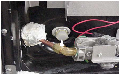
Water Heater Drain Plug (Remove with socket)
