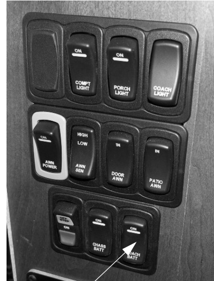
House/Coach Battery Disconnect Switch (Located near entrance door) -Typical View
