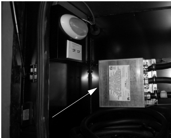
Automatic Power Transfer Box (Located inside or behind utility compartment) -Typical Installation
