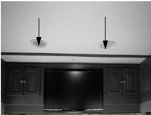
Supply/Return Air Vents (Located throughout the ceiling of the coach) -Typical View
