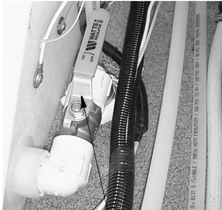
Water Tank Drain Valve (Typical)
