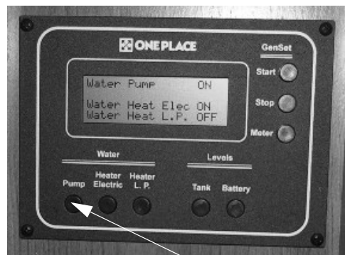
Water Pump Switch
