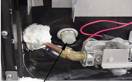
Water Heater Drain Plug (Remove with socket)
