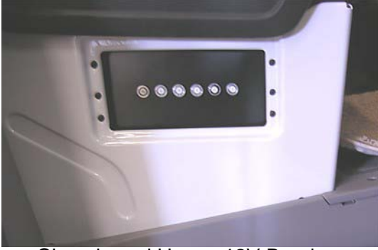
Chassis and House 12V Breakers (Located on side of passenger seat base toward door) * Shown with cover removed -Typical View
