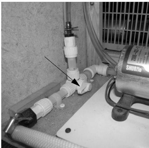
Winterization Valve -Typical View
