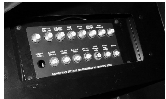
Chassis and House 12V Breakers -Shown with cover removed
