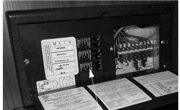
120-Volt Circuit Breakers -Typical View
