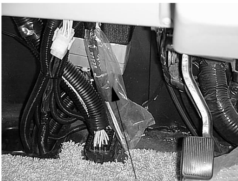
CB Power Wires (in plastic sheath)
