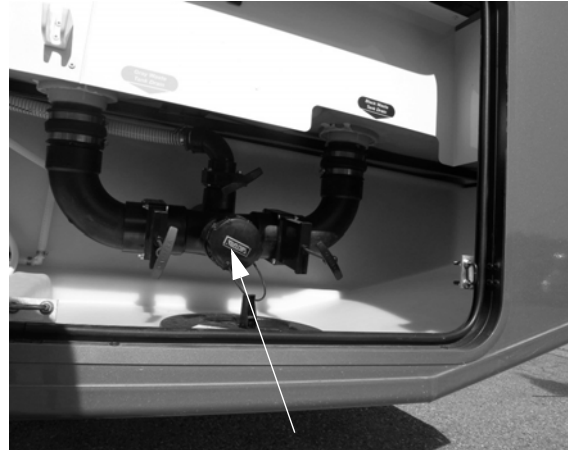
Sewage Drain Outlet (Located in water service center) -Typical View
