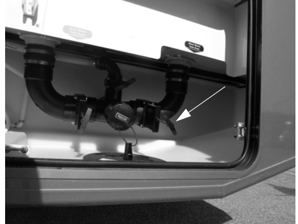
Black Waste Tank Drain Valve (Rear) (Located in water service center) -Typical View
