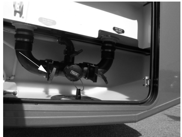
Gray Waste Tank Drain Valve (Located in water service center) -Typical View
