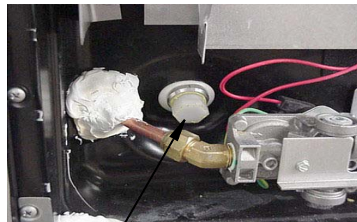
Water Heater Drain Plug (Remove with socket)
