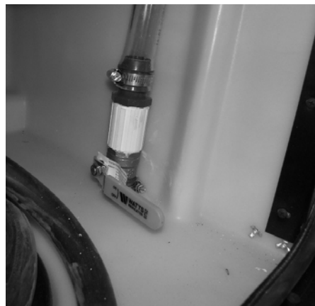
Water Tank Drain Valve -Typical installation shown
