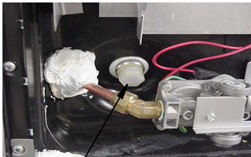
Water Heater Drain Plug (Remove with socket)
