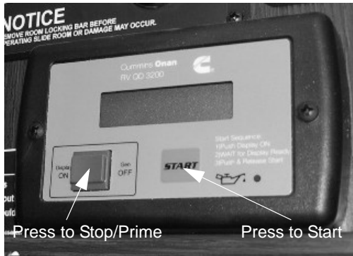
Diesel Generator Start/Stop Buttons (Located near monitor panel) -Typical View
