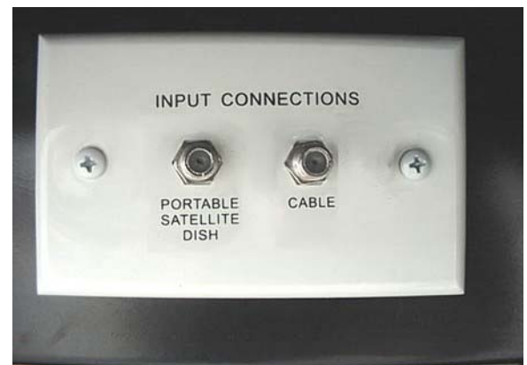
Exterior Cable TV and Satellite Connections (Located in shoreline or utility compartment, depending on model)
