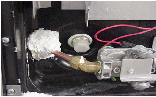
Water Heater Drain Plug (Remove with socket)
