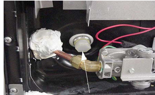
Water Heater Drain Plug (Remove with socket)
