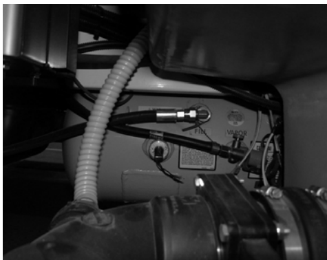
Propane Gas Tank (Located under center of coach) -Typical View
