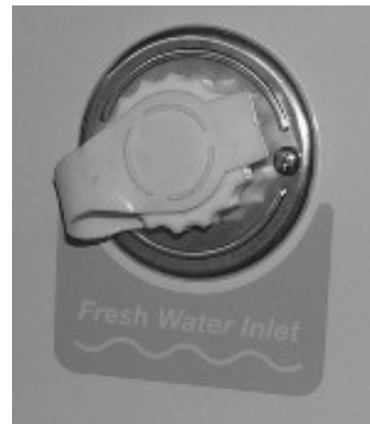
Fresh (City) Water Connection (Fresh Water Inlet)
