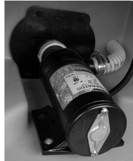
Waste Pump (Located behind removable panel in water service center) -Typical View
