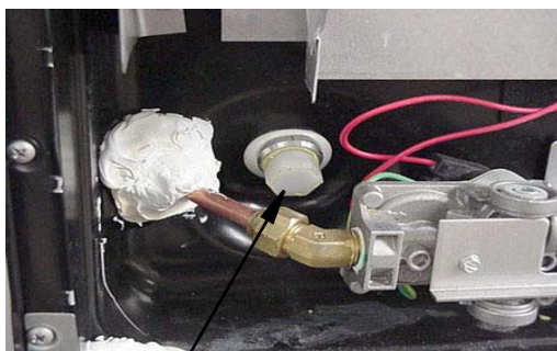
Water Heater Drain Plug (Remove with socket)
