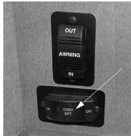
House/Coach Battery Disconnect Switch (Located near entrance door) -Typical View
