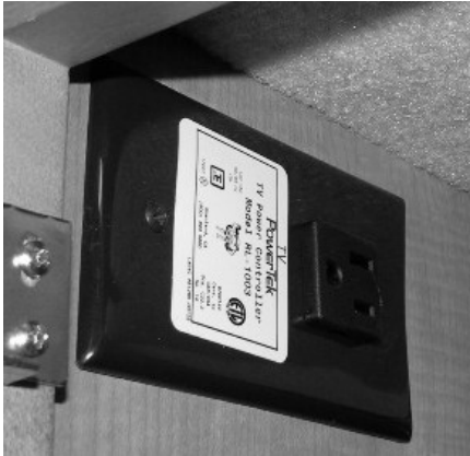
Front TV Ignition Switch Interlock -Typical View
