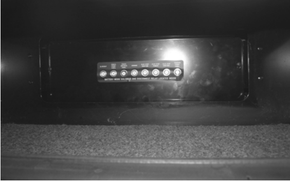
Automotive Chassis and House 12-Volt Circuit Breakers (Located inside passenger compartment) -Typical View
