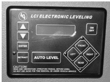
Leveling System Control Panel (Located on dash)
