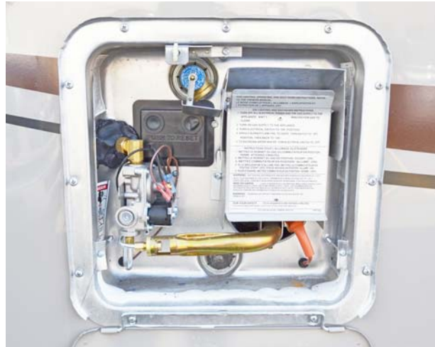
Water Heater Exterior Service Access
