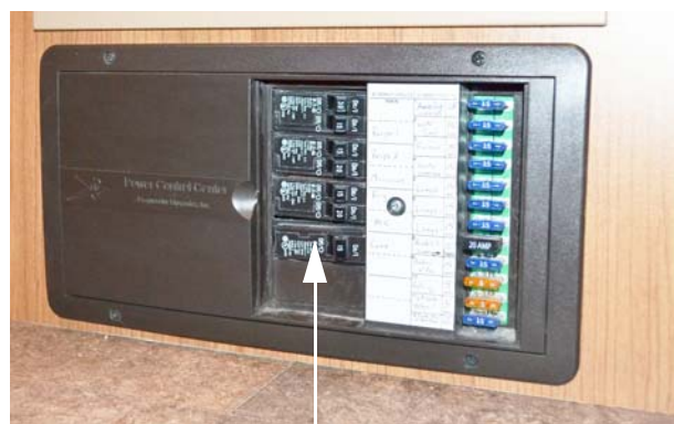
120-Volt Circuit Breakers -Typical View
