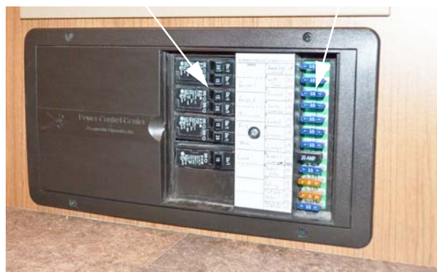
Power Center (Converter) -Typical View
