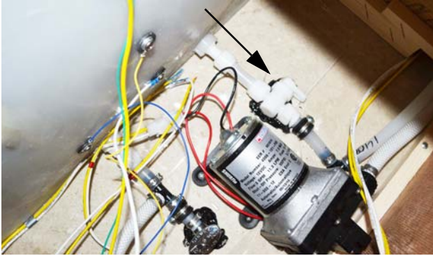
Waterline Drain Valve -Typical View
