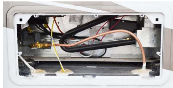
Refrigerator Access Compartment -Typical View
