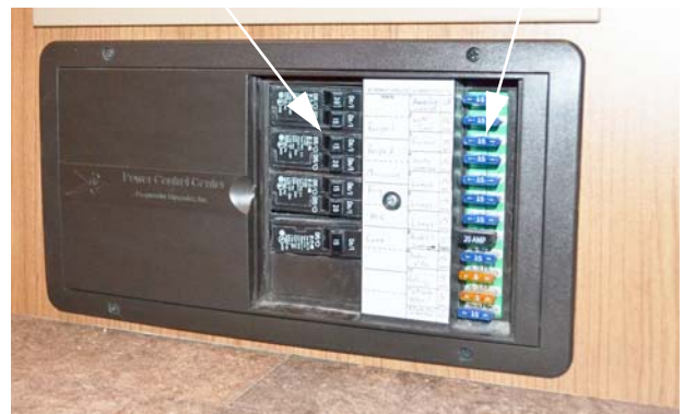
Power Center (Converter) -Typical View
