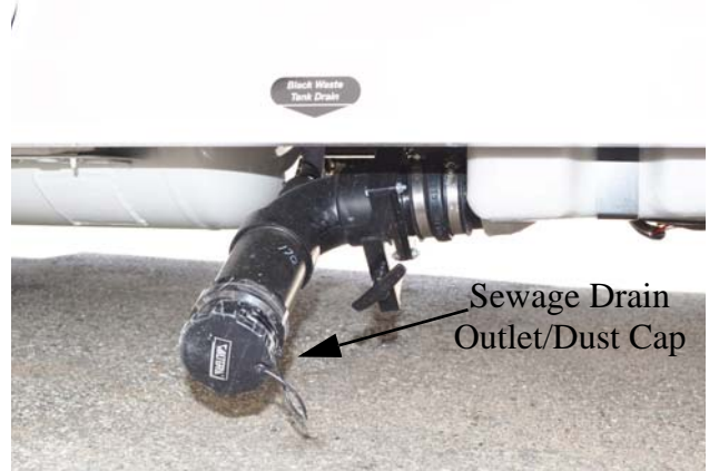
Sewage Drain Outlet (Located beneath coach on mid-driver side) -Typical View
