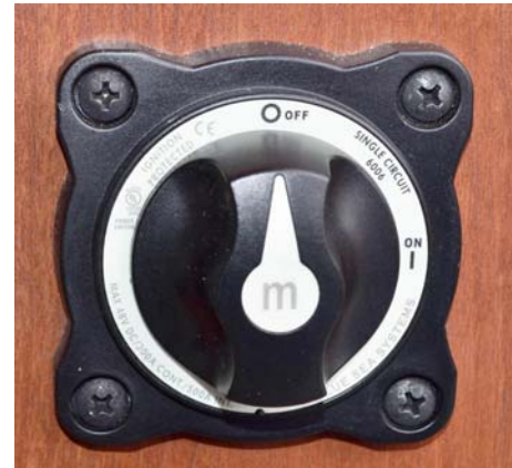
House/Coach Battery Disconnect Switch (Located near entrance door) -Typical View
