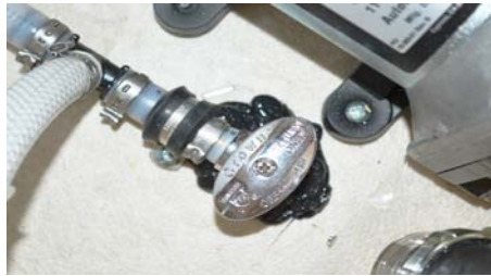
Water Tank Drain Valve (Typical)
