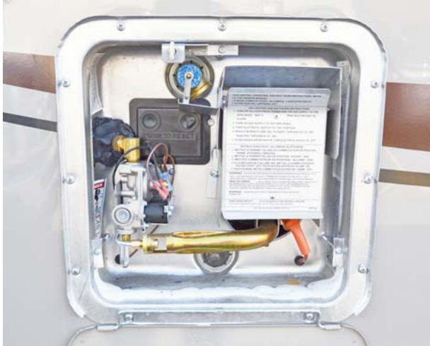
Water Heater Exterior Service Access
