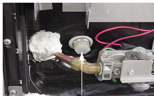
Water Heater Drain Plug (Remove with socket)
