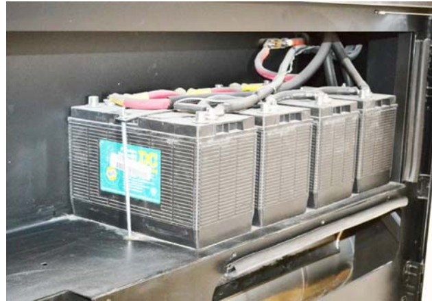
House/Coach Batteries -Typical View
