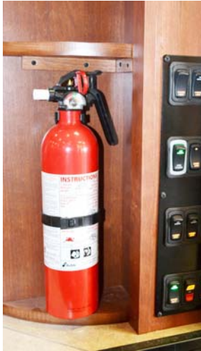
Fire Extinguisher (Located near entrance door) -Typical installation shown
