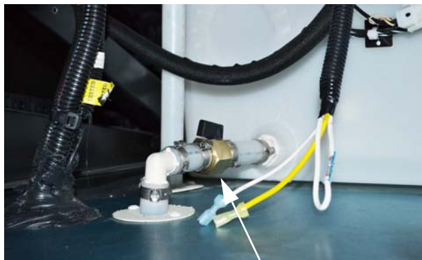
Water Tank Drain Valve (Located in second driver side compartment) *Model 34T shown
