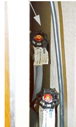
Water Supply Faucets (Located behind access panel within wardrobe) *Model 34T
