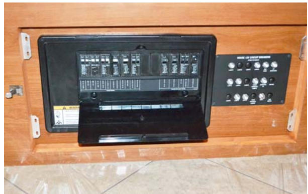
House Circuit Breakers -Typical Installation
