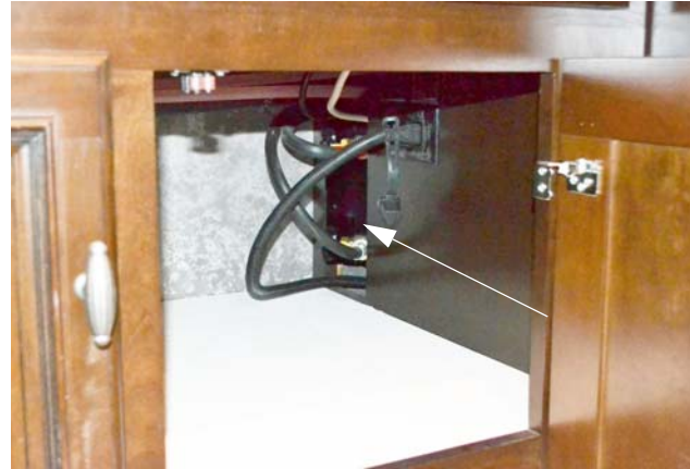
Water Supply Faucets (Located below lavatory cabinet)
