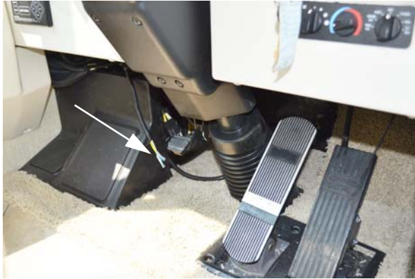
CB Power Wires -Typical View
