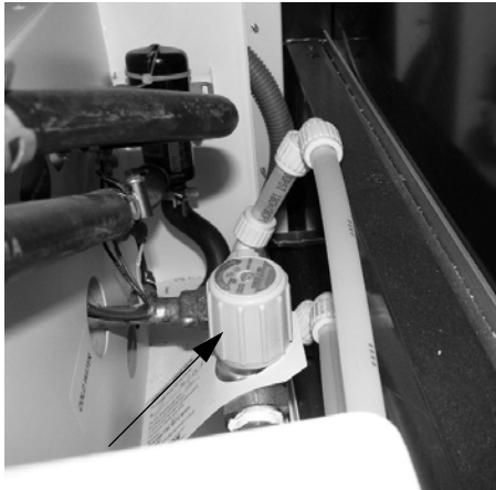
Hydronic Heating System Tempering Valve (Located on back side of the Aqua-Hot unit)
