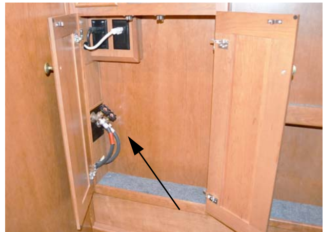
Water Supply Faucets (Located inside bathroom wardrobe cabinet)
