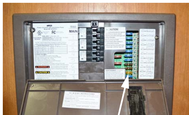
House 12-Volt Fuses (Located on the right-hand side of the Power Converter) (Models 27N and 30T) -Typical View
