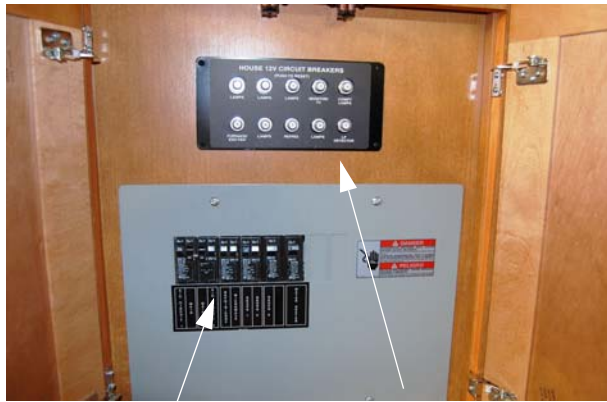
120-Volt House Circuit Breakers
