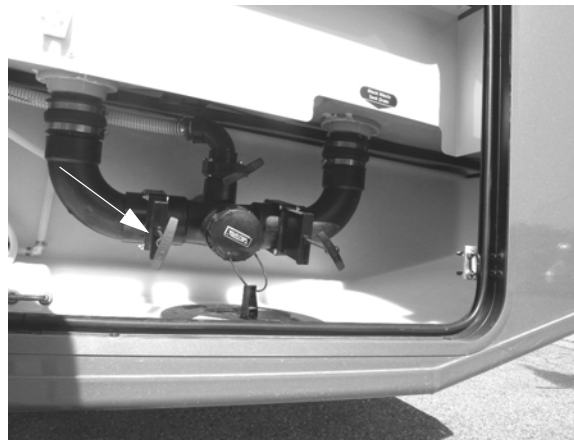
Gray Waste Tank Drain Valve (Located in water service center) -Typical View
