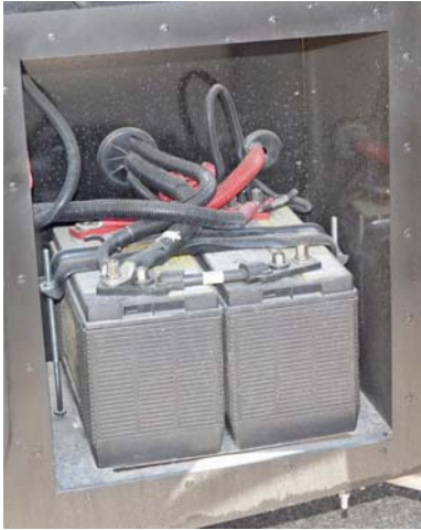
Chassis Batteries (Located behind a rear driver side exterior door) -Typical View
