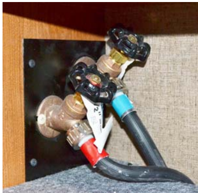
Water Supply Faucets -Typical View
