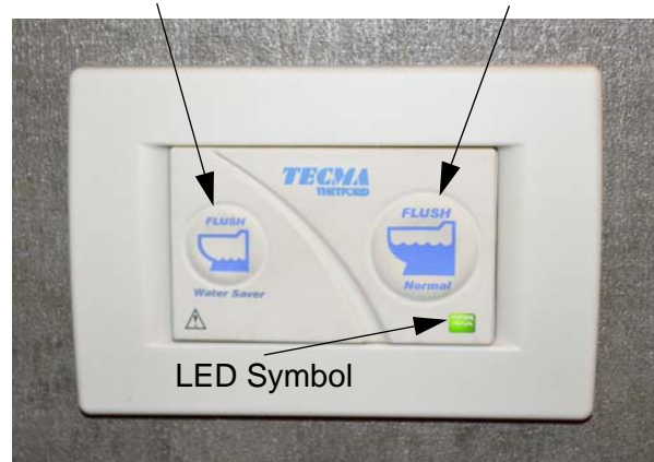
LED Symbol Wall Switch/Controller (Located on wall near toilet)
