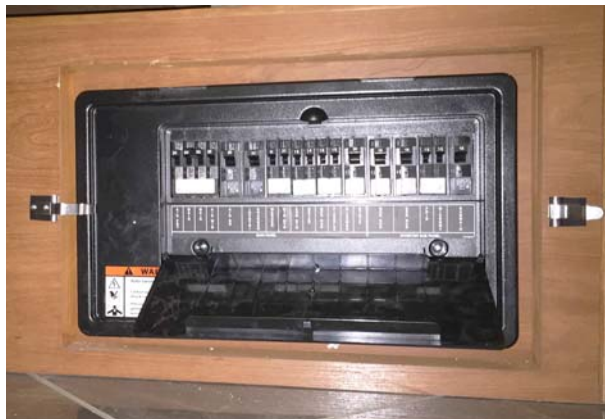
House Circuit Breakers -Typical Installation
