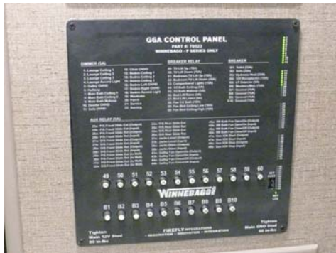
House Circuit Breakers -Typical View
