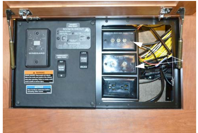
Interior Connections for Satellite Dish (Located in the overhead compartment above the driver seat)
