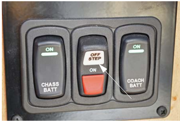
Entry Step Switch (Located near the entrance door) -Typical View
