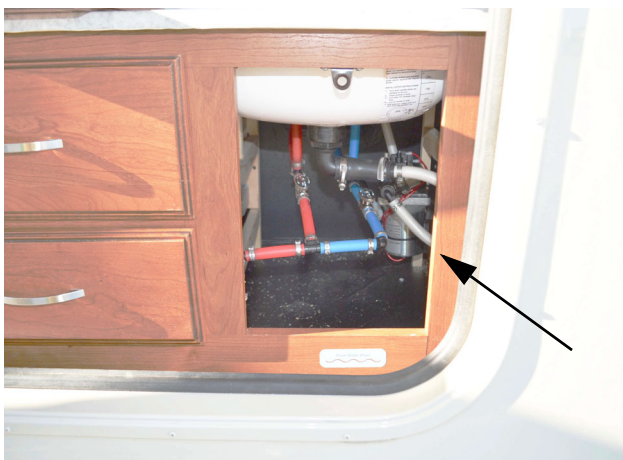
Exterior Sink Pump (Located in the passenger side compartment behind rear axle) -Typical View
