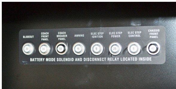
Automotive Chassis and House 12-Volt Circuit Breakers (Located inside passenger compartment) -Typical View
