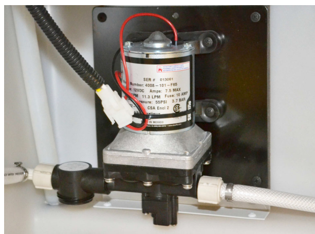
Water Pump -Typical View
