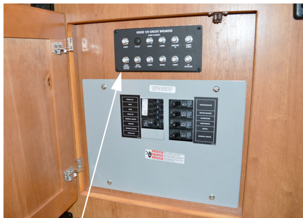
House 12-Volt Circuit Breakers
