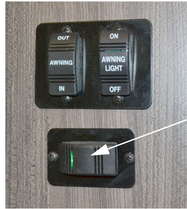
Accent LED Running Board Light Switch (Located near sliding door) -Typical View
