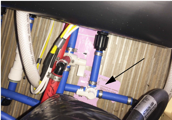
Winterization Valve 2 (See “Water System Drain Valve Locations” chart at the end of this section for location on your model) *Model 59KL shown
