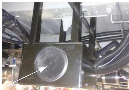
Waste Pump Enclosure (Located beneath motorhome)
