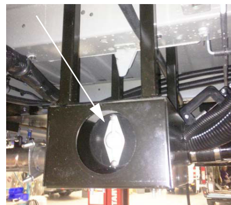
Waste Pump (Located beneath motorhome)
