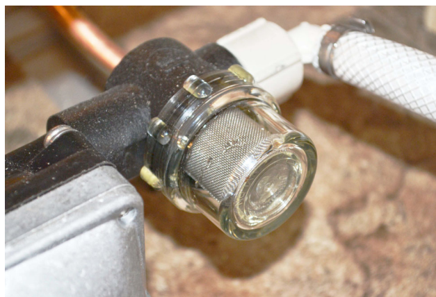
Shower Filter Screen (Located beneath galley cabinet access panel) -Typical View
