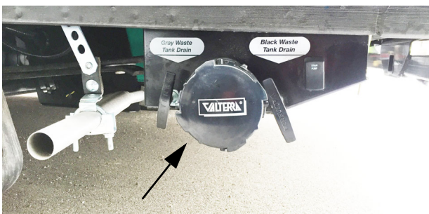
Sewage Drain Outlet (Located beneath motorhome) *Model 59GL
