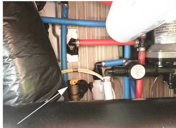
Water Heater Drain (Yellow) Valve
