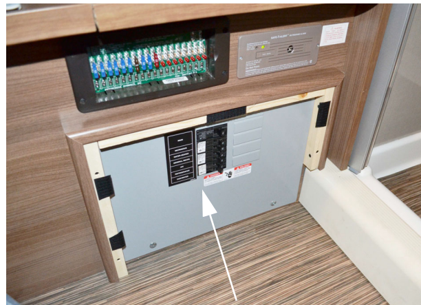
120-Volt Circuit Breakers -Typical View
