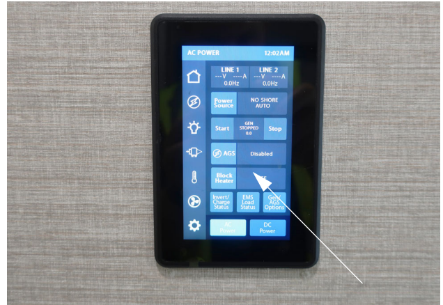
Diesel Engine Heater Switch (Located on multiplex monitor panel)
