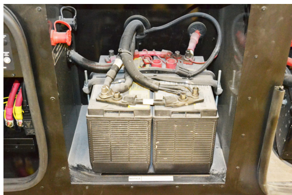
Chassis Batteries -Typical View
