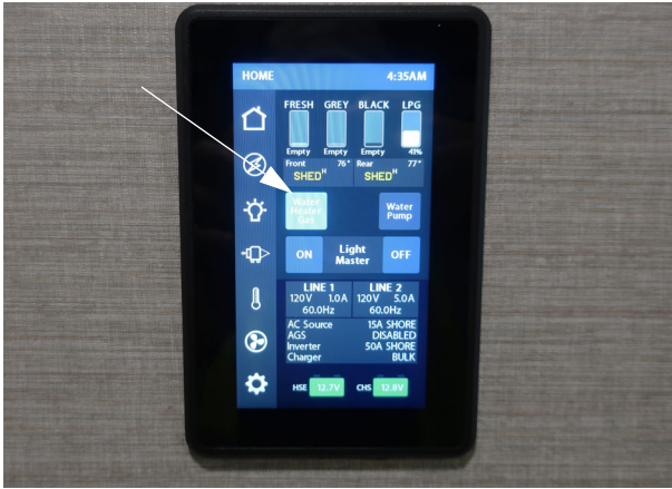
Water Heater Switch “HOME” Screen (Located on Multiplex Monitor Panel)
