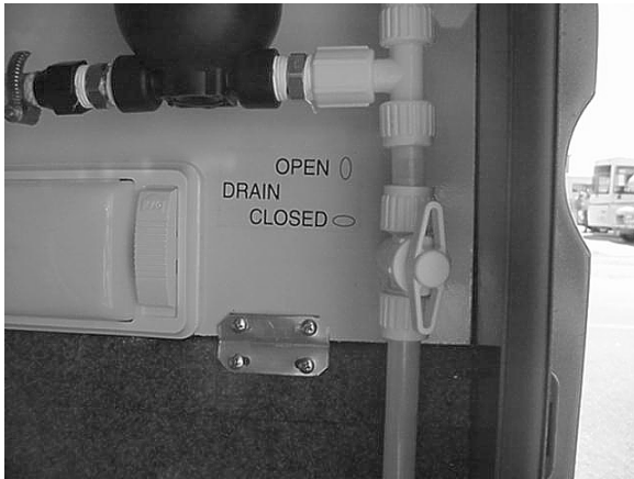
Water Line Drain Valve
