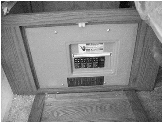
110-Volt Breaker Panel below Bedroom Wardrobe
