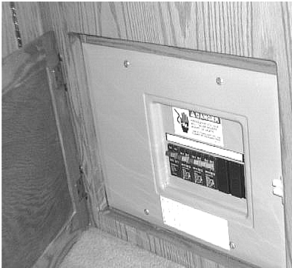
House 110-Volt Breaker Panel near Entrance Step
