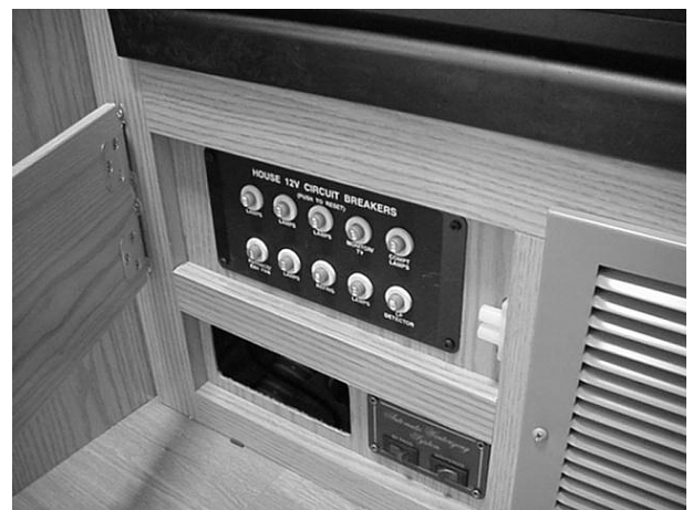
House 12-Volt Breaker Panel
