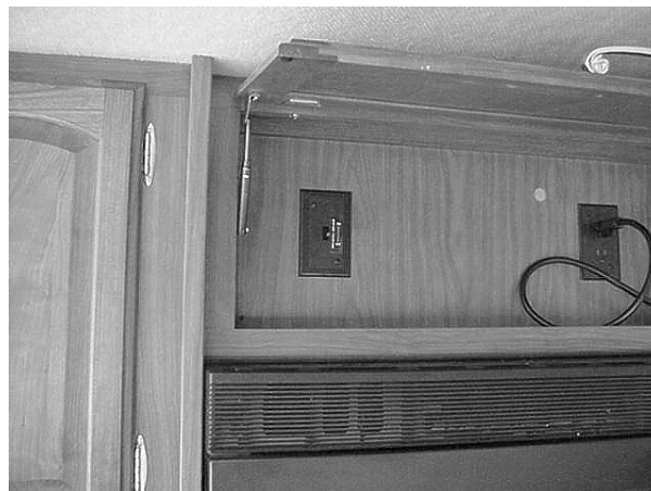
Electric Water Heater Switch (above microwave)
