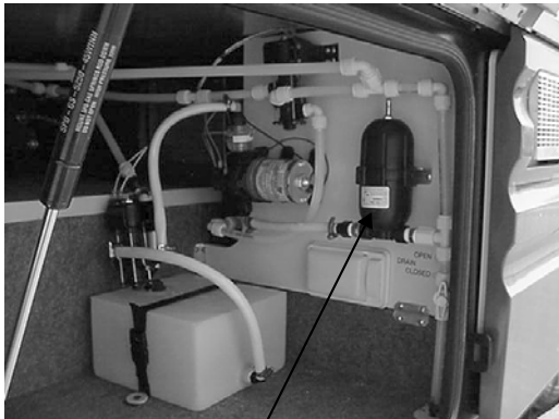
Water Pressure Accumulator Tank
