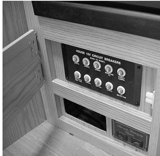
House 12-Volt Breakers
