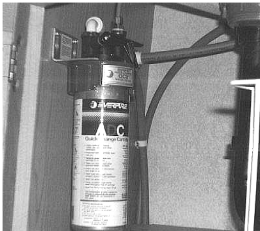
Water Filter Assembly - Below Galley Sink
