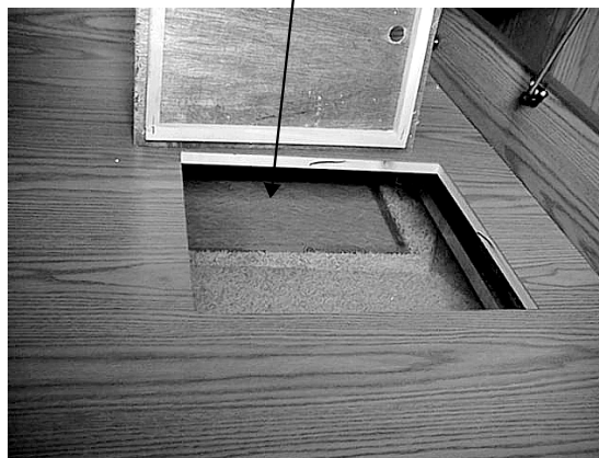
Air Conditioner Filter (Beneath bed)
