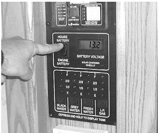
Battery Voltage Check One Place Panel
