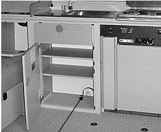
Water Line Drain Valve
