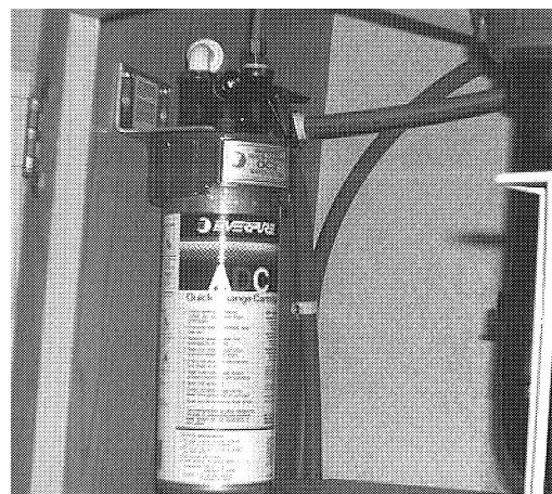
Water Filter Assembly - Below Galley Sink
