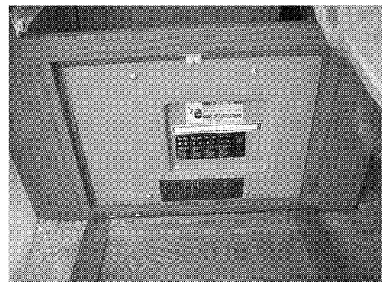
110-Volt Breaker Panel below Bedroom Wardrobe
