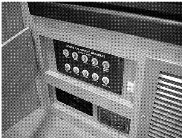
House 12-Volt Breaker Panel
