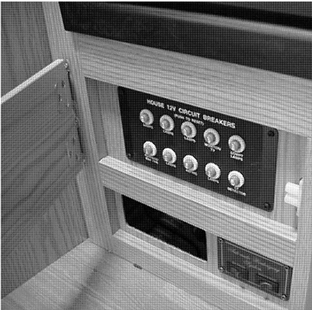
House 12-Volt Breakers
