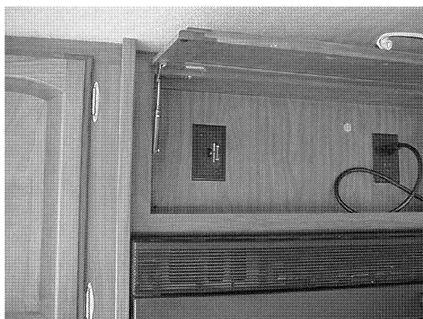
Electric Water Heater Switch (above microwave)
