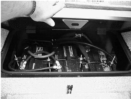
Lift step to access batteries
