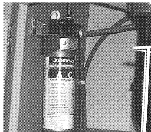
Water Filter Assembly - Below Galley Sink
