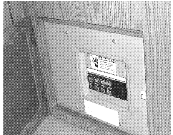
House 110-Volt Breaker Panel near Entrance Step
