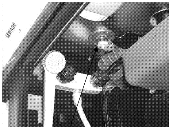
City Water Connection
