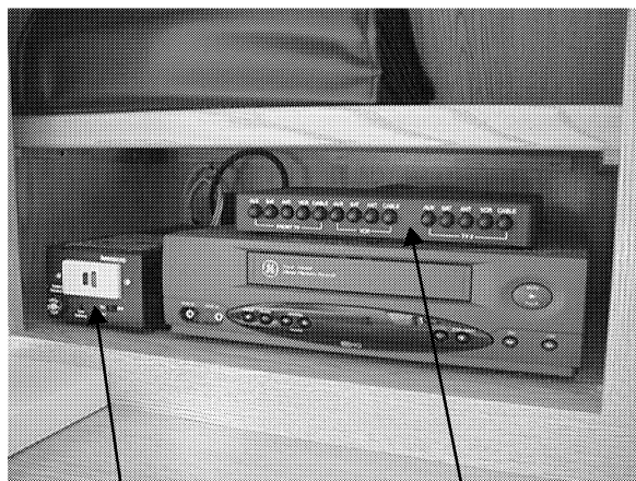
DC/AC Inverter Video Selector System
