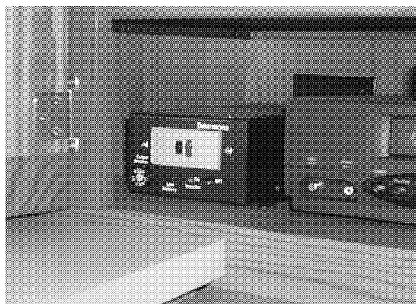
DC-AC Voltage Inverter in Video Center
