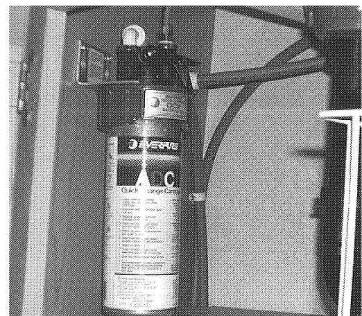
Water Filter Assembly - Below Galley Sink
