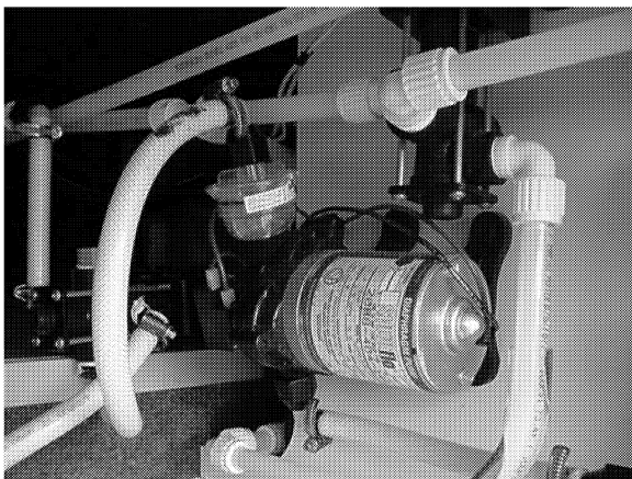
Water Pump in right front compartment
