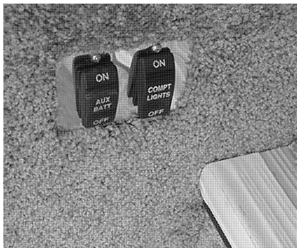
Aux. Batt. Switch (Near entrance door)
