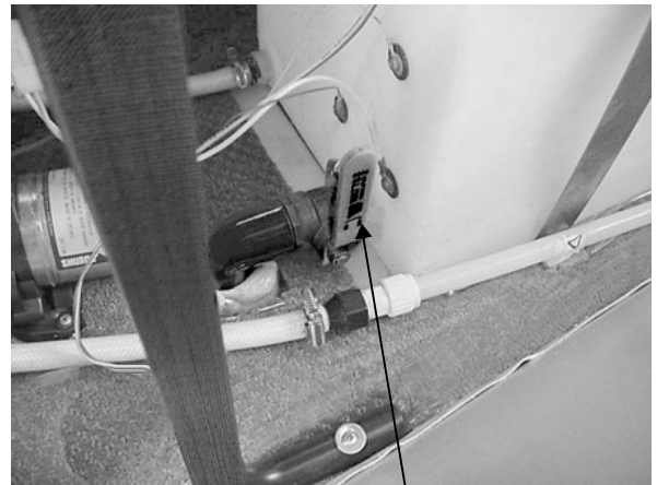
Water Tank Drain Valve
