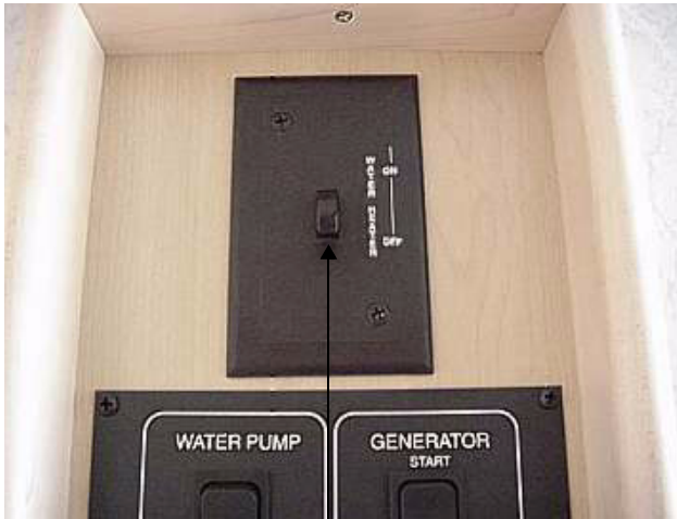
Electric Water Heater Switch above One Place Panel
