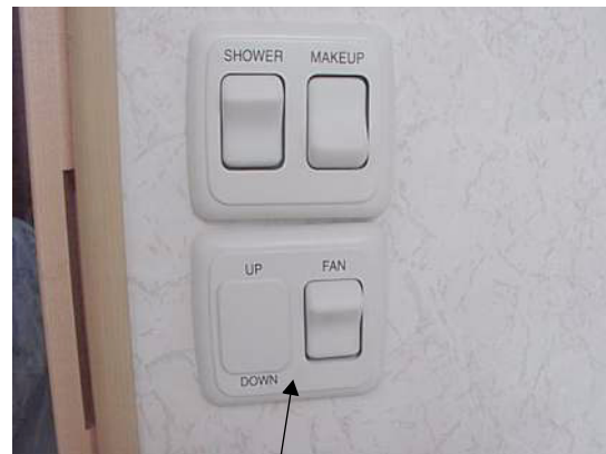
Bath Vent Controls
