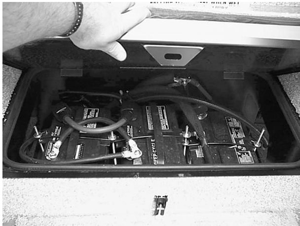
Lift step to access batteries
