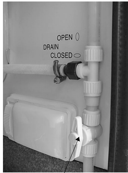
Water Line Drain Valve
