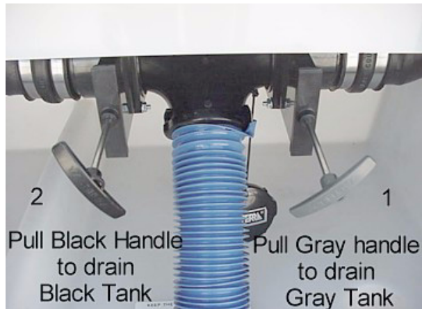
Holding Tank Valves (Typical)
