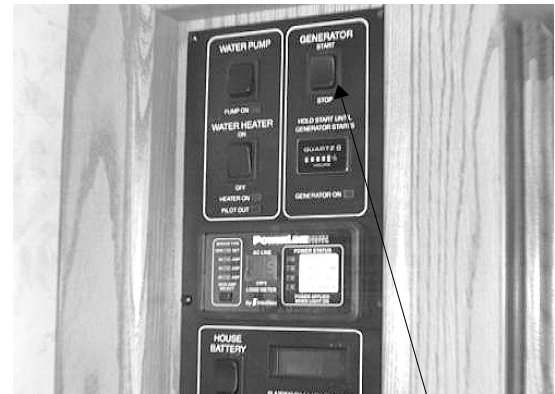
Generator Switch and Hourmeter
