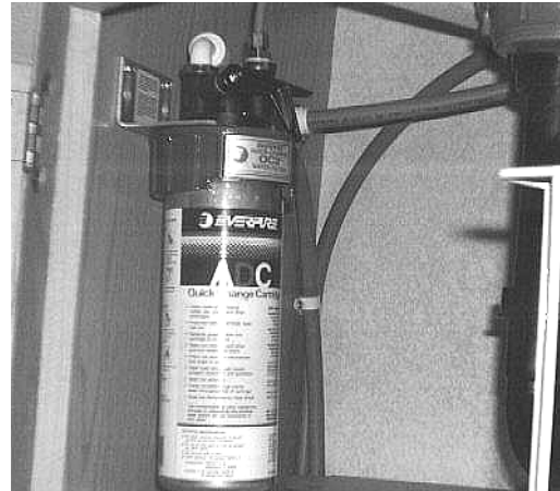
Water Filter Assembly - Below Galley Sink
