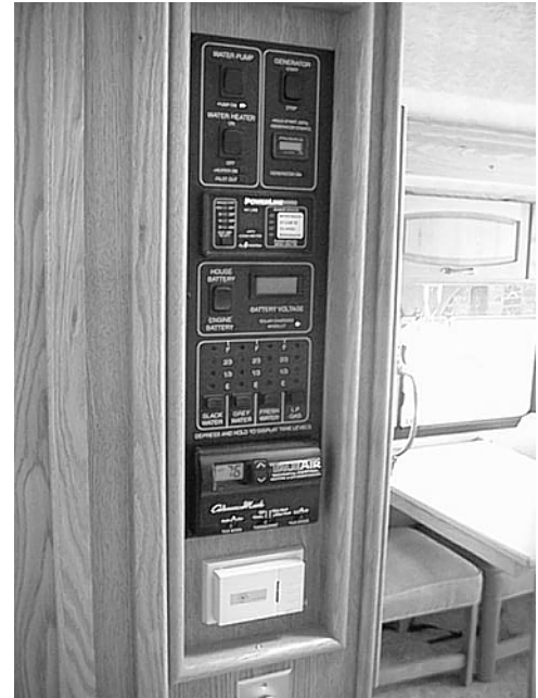
One Place Monitor Panel
