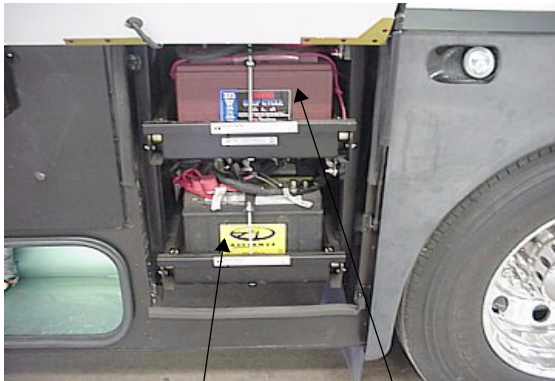
Chassis Batteries House Batteries
