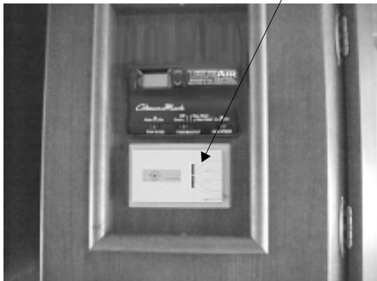
Power Ventilator Thermostat - Galley
