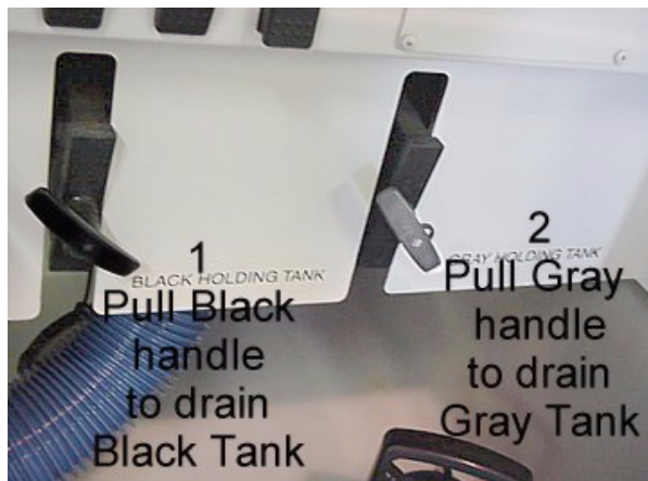
Holding Tank Valves (Typical)
