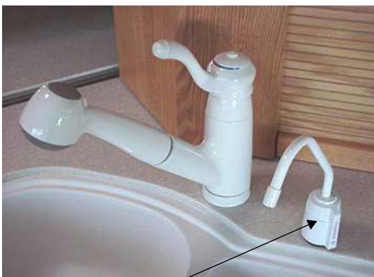
Filtered Water Faucet (Typical)
