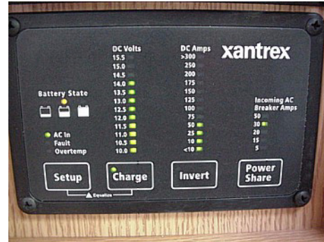
Inverter Charger Control Panel
