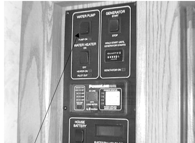
Water Pump Switch
