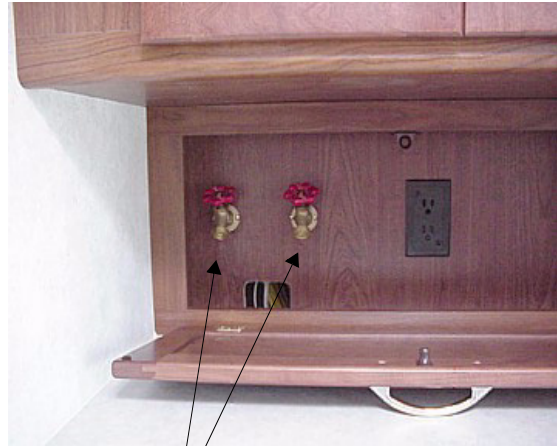
Water Supply Faucets Typical
