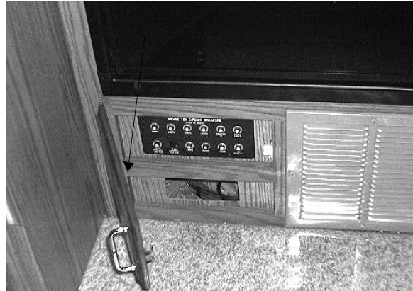
House 12-Volt Circuit Breaker Panel
