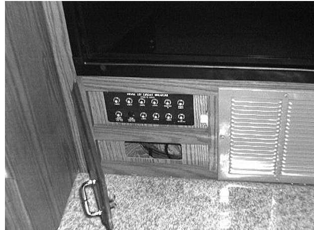
House 12V Breakers (below refrigerator)
