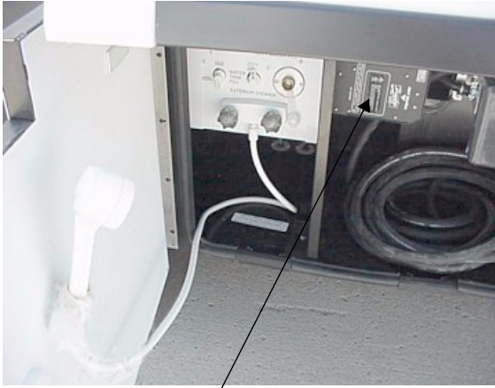
Inverter Charger Unit Location
