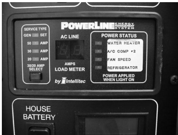
EMS Display on OnePlace Monitor Panel
