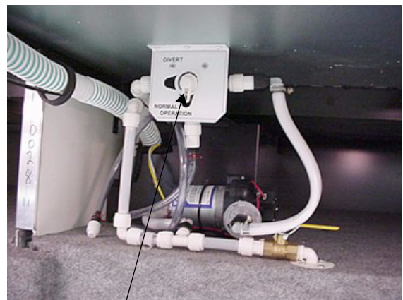
Water Heater By-Pass Valve
