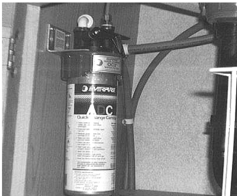
Water Filter Assembly - Below Galley Sink
