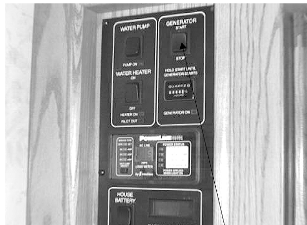
Generator Switch and Hourmeter
