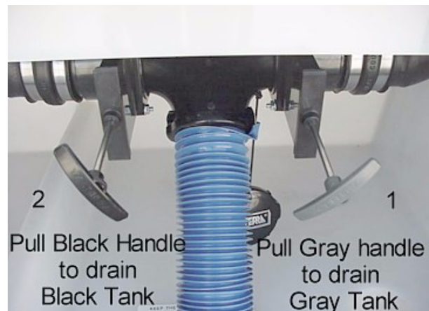
Holding Tank Valves (Typical)
