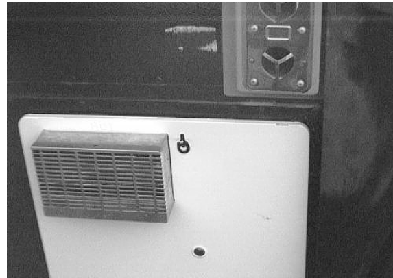
Water Heater Service Access Panel
