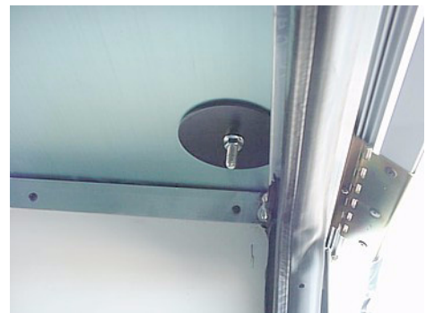
Bolt is visible on ceiling of exterior storage compartment below dinette.
