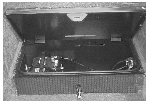
House Battery in Top Entrance Step
