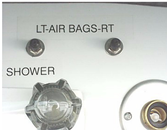
Rear Helper Spring Air Valves located inside water center
