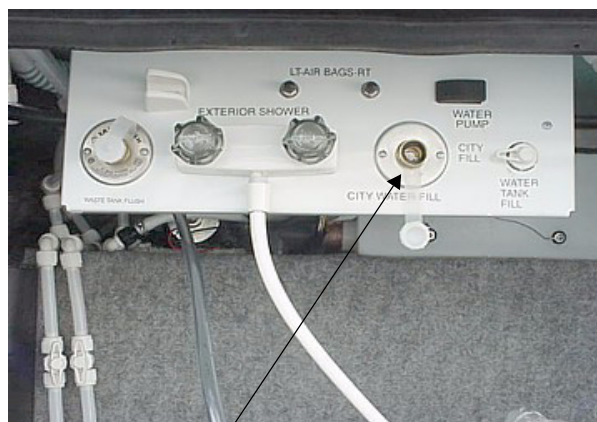
City Water Connection
