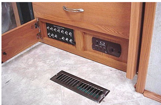
House 12V Breakers (below refrigerator)
