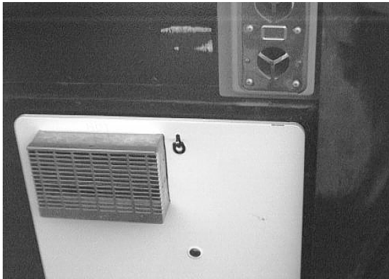
Water Heater Service Access Panel
