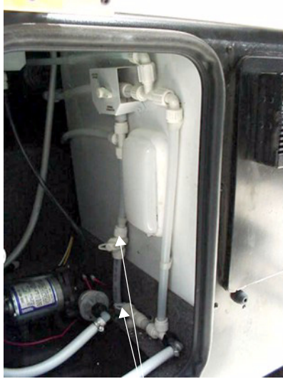
Water Line Drain Valves
