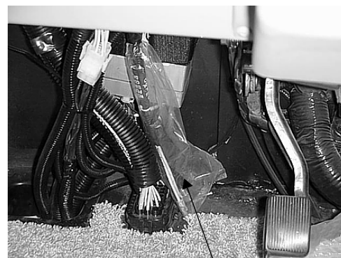
CB Power Wires (in plastic sheath)
