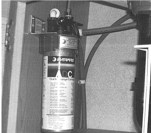
Water Filter Assembly - Below Galley Sink
