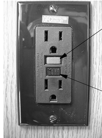
GFCI Outlet (Ground Fault Protector)
