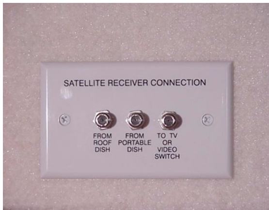
Interior Connection for Satellite Dishes (in front video center cabinet)
