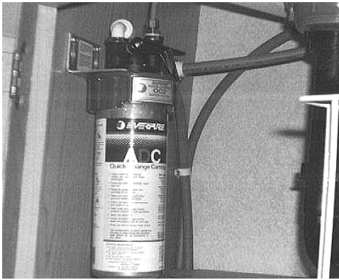
Water Filter Assembly - Below Galley Sink
