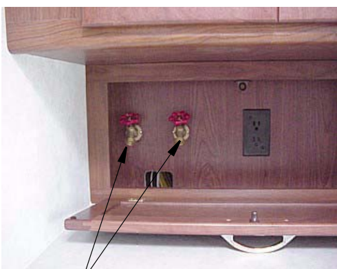
Water Supply Faucets -typical
