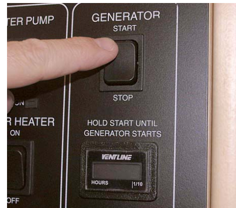
Generator Switch and Hourmeter on monitor panel
