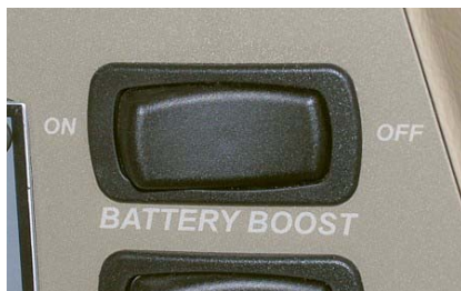
Battery Boost Switch
