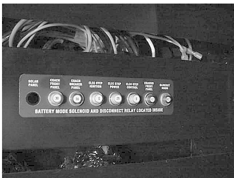
Auto Chassis 12-Volt Circuit Breaker Panel (cover removed)
