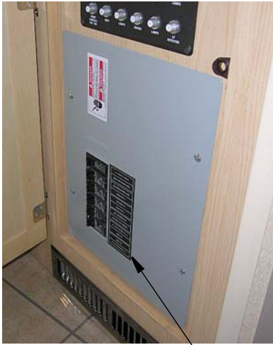
120-Volt House Circuit Breakers - typical
