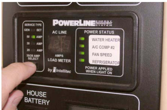
PowerLine EMS Display on Monitor Panel - typical
