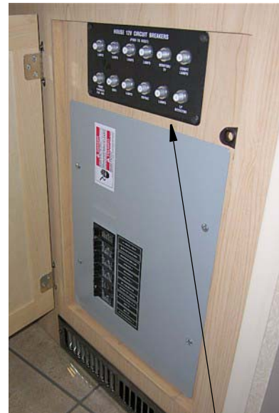
House 12-Volt Circuit Breaker Panel
