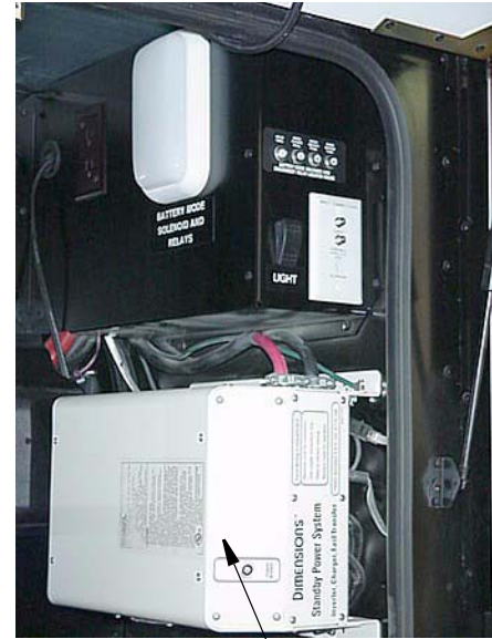
Inverter Charger Unit Location (in utility compartment)
