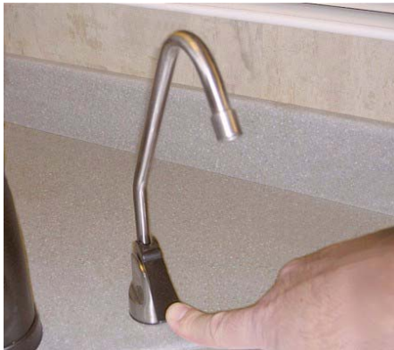
Filtered Water Faucet
