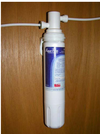
Water Filter Assembly (Located below Galley Sink)
