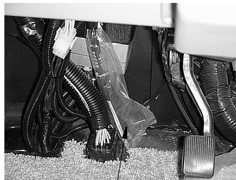
CB Power Wires (in plastic sheath) Typical view - your coach may differ slightly
