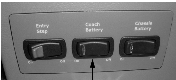
Aux. Battery Disconnect Switch (Near Entrance Door)
