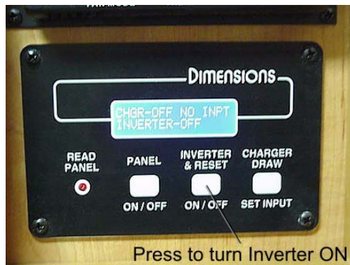
Inverter/Charger Control Panel
