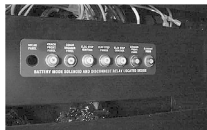
Chassis and House 12V Breakers (cover off)
