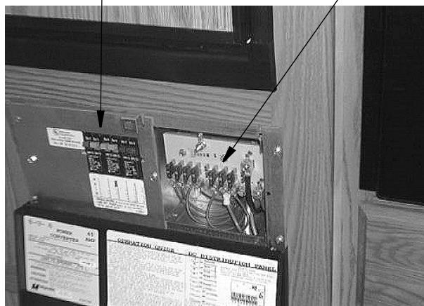
Power Center (Converter)
