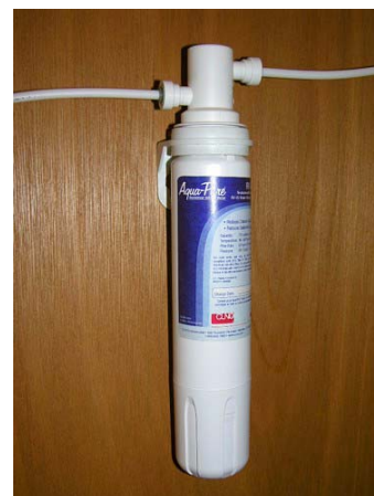
Water Filter Assembly below Galley Sink
