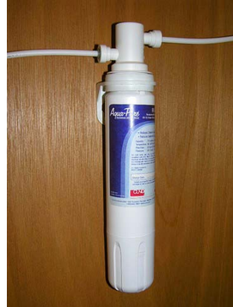
Water Filter Assembly below Galley Sink
