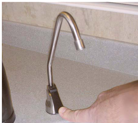
Filtered Water Faucet
