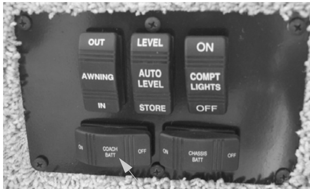
Auxiliary Battery Switch - Typical (Near Entrance Door)
