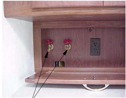
Water Supply Faucets - Typical
