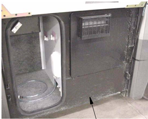
Water Pump Access Panel (typical)
