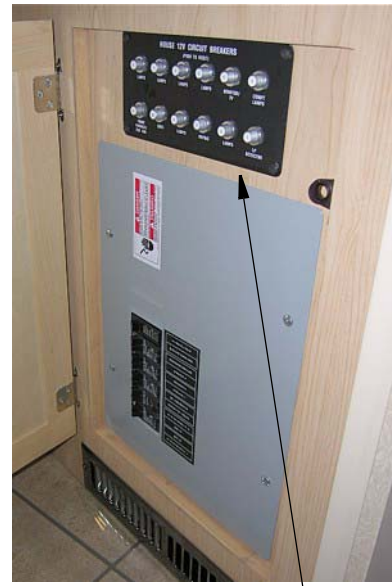
House 12-Volt Circuit Breaker Panel
