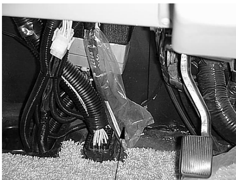
CB Power Wires (in plastic sheath) typical view - your coach may differ slightly
