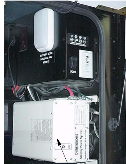
Inverter Charger Unit Location (in utility compartment)
