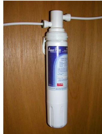
Water Filter Assembly below Galley Sink
