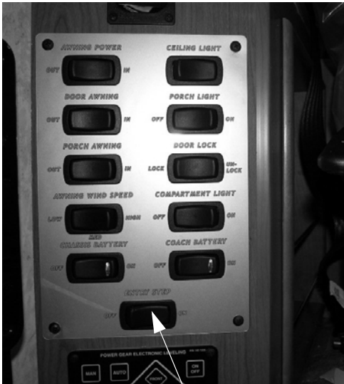
Entry Step Switch - Typical (Located near the entrance door)
