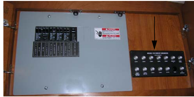
House 12-Volt Circuit Breaker Panel
