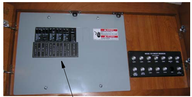
House 120-Volt AC Circuit Breaker Panel
