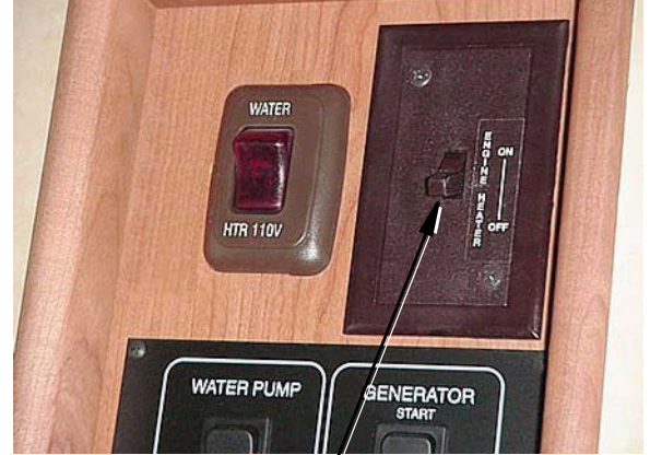
Diesel Engine Heater Switch (Typical)
