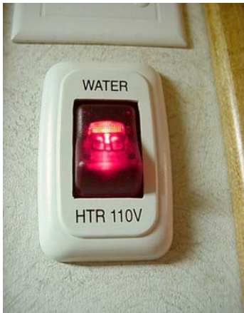
Electric Water Heater Switch (typically located near Systems Monitor Panel)
