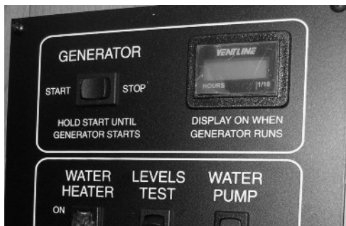
Generator Switch and Hourmeter on monitor panel
