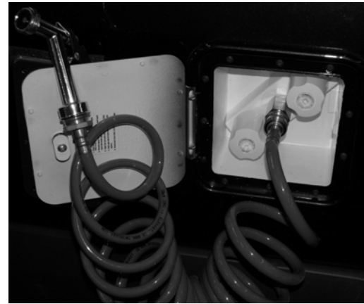
Exterior Shower/Wash Station (Typical)
